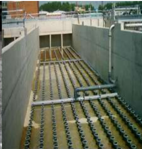
Sub Surface Aeration
